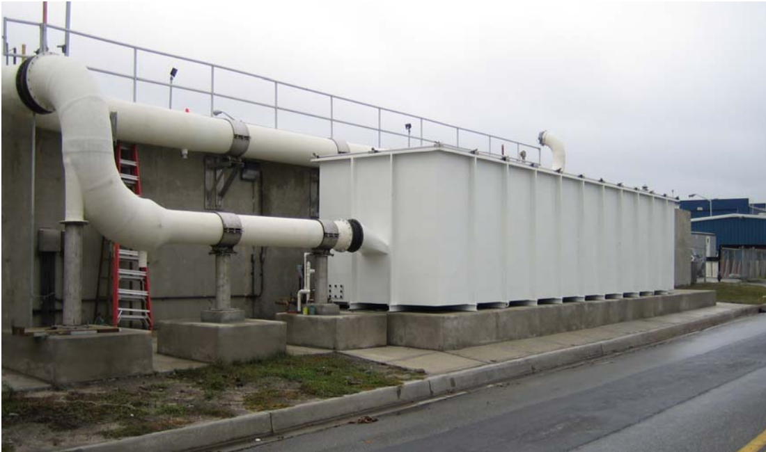
Figure 2: An Integrated Modular Stainless Steel Biofilter Vessel (Photo courtesy of BIOREM Technologies Inc.)
