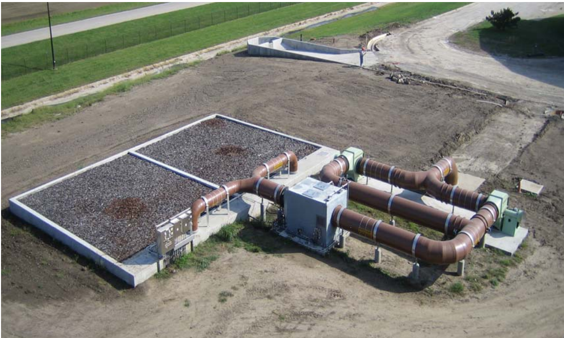
Figure 3: An Open-top, Custom, Field-erected, In-ground Concrete Biofilter (Photo courtesy of BIOREM Technologies Inc.)
