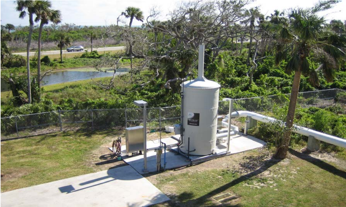
Figure 6: A Modular FRP Biotrickling Filter
